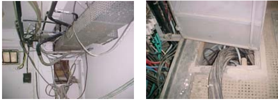
Transforming Cabins before restoration
