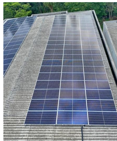
Photovoltaic plant installed in the Suzano Auxiliary Hospital
